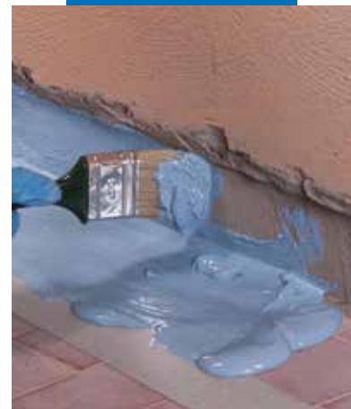
Application of Mapelastac AquaDefense by brush between floor and wall before applying Mapeband
